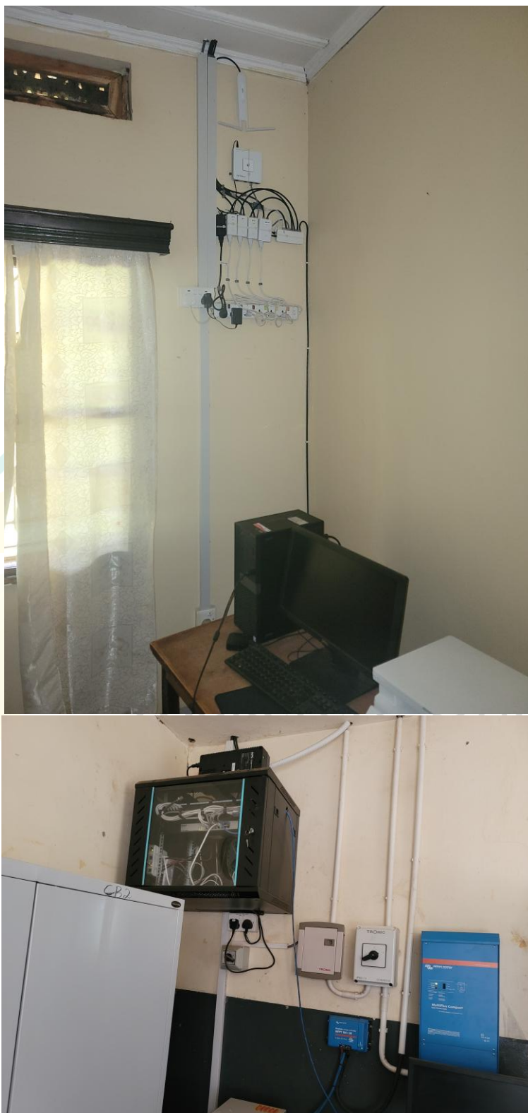
Part of the Network infrastructure setup at Buikwe HC III in Buikwe district
